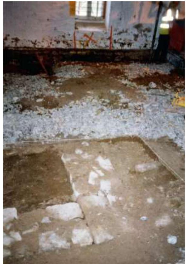
(right) The foundation walls of the 1830s Malthouse, revealed below the 1890s floor.
